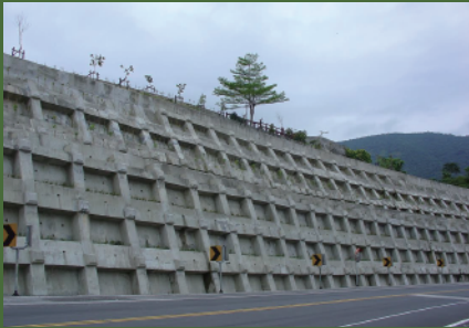
Hualien-Taitung Coastal Highway Slope Drainage, Taiwan
