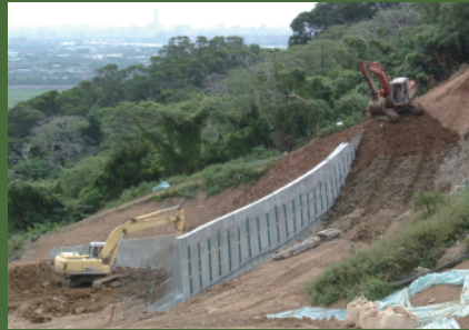
Taipei National University of the Arts Collapse Recovery, Taiwan
