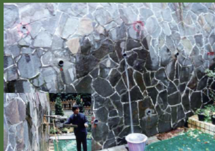
Wenquan Road Retaining Wall Drainage, Taiwan
